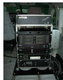
LIDAR Control Rack
