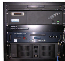
Camera Control Rack
