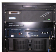
Camera Control Rack
